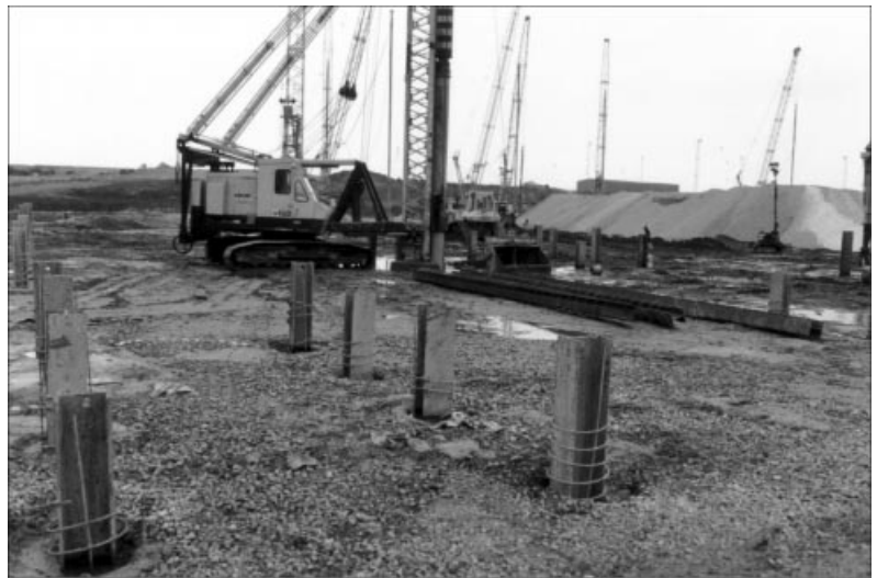
Fig. 18. Detail of 480 mm diameter cast-in-place driven piles showing the UBP steel sections and shear helical
