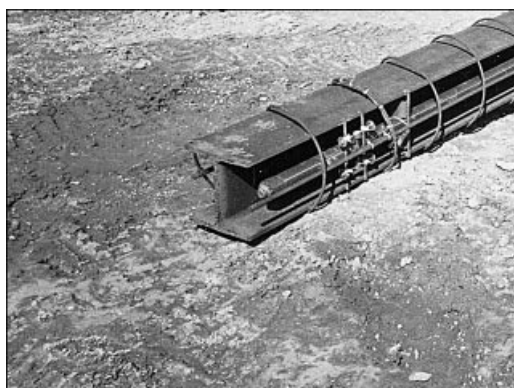
Fig. 21. Preliminary test pile reinforcement fitted with strain gauges, inclinometer access tubes and extensometer bars
