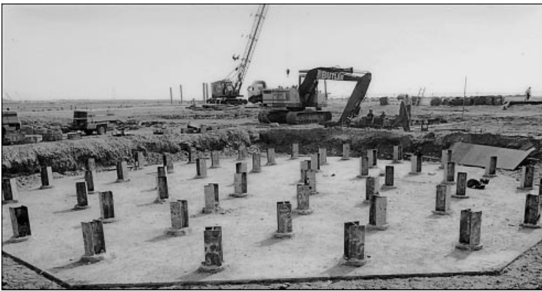
Fig. 27. Foundation footprint to a storage tank showing the pile heads and steel UBP sections
